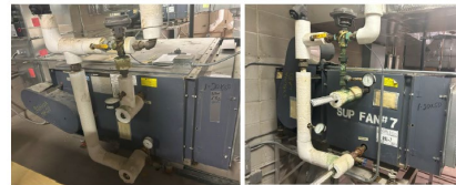
Air handling units serving multiple areas. System age 34 years. Life expectancy 25-30 years.
